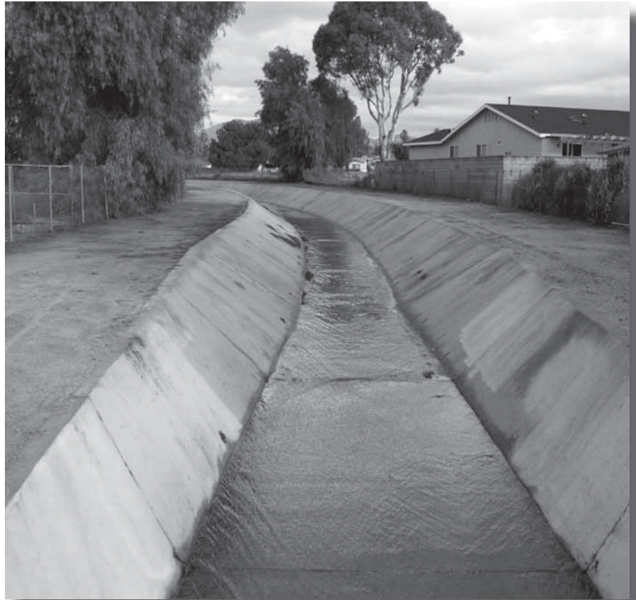
Under the new permit there will be fewer concrete channels such as this one used to move rainwater off sites quickly. Water flows at high velocity through these channels and washes out downstream waterways.
